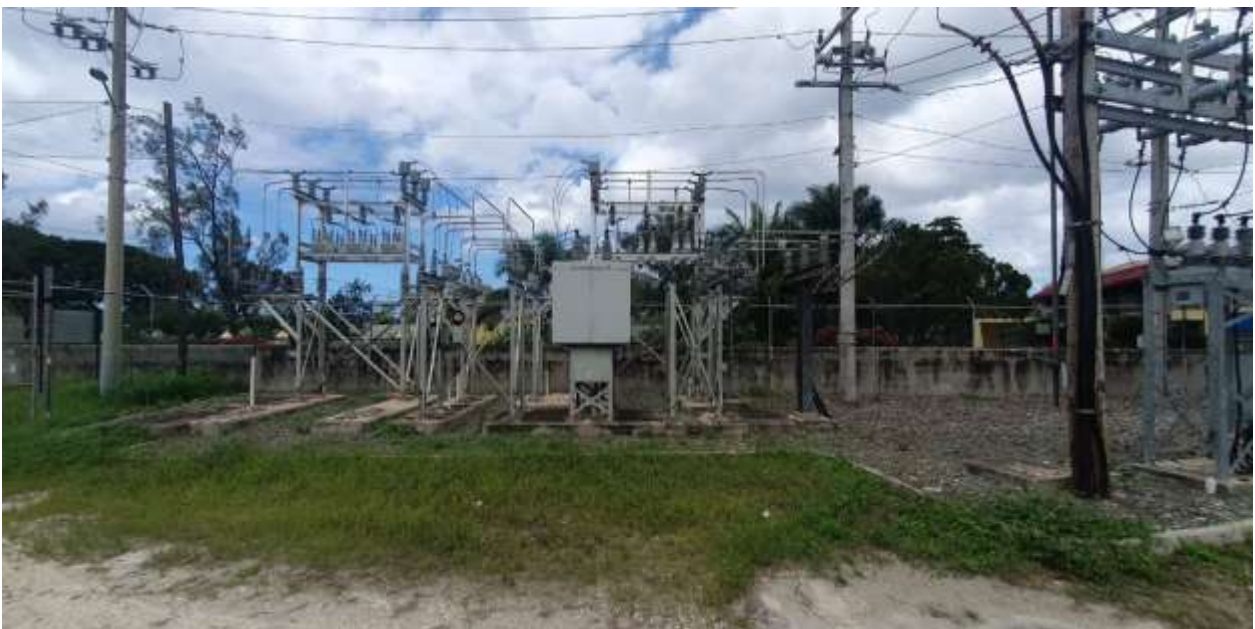
Figure 3: Cardiff Hall Substation
